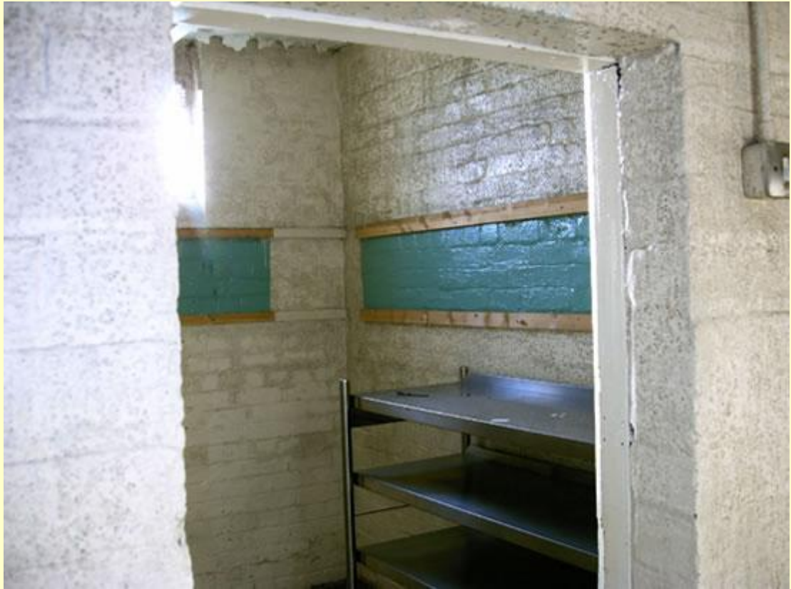
This is one of the solitary cells in the detention block, which was latterly used as stores.
