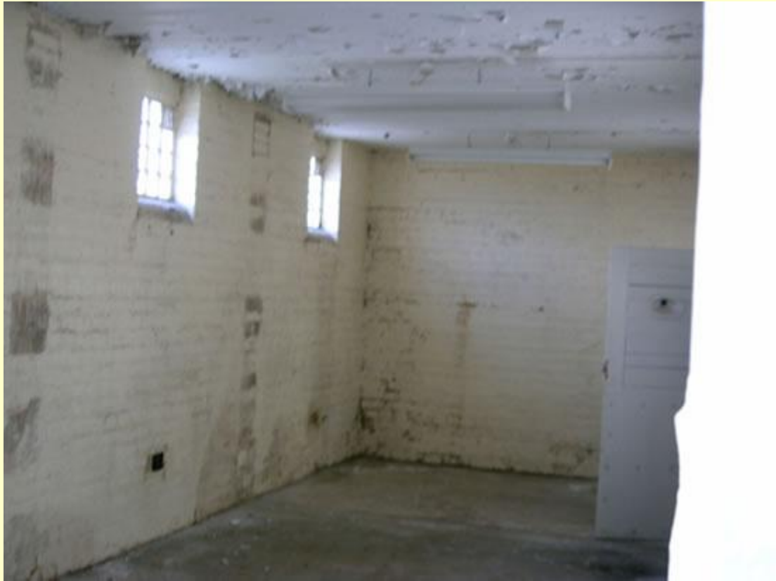
This room was created out of three former cells, and their respective dimensions can be gauged from the marks on the walls.
